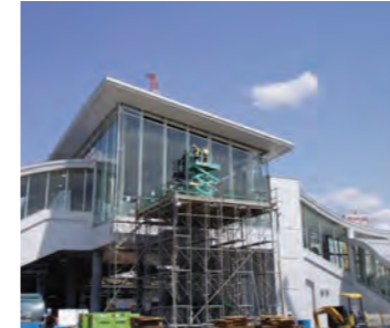
New construction of the Matsumoto Station West Entrance on the JR Shinonoi Line
